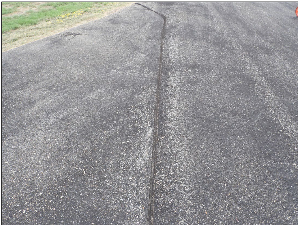
TW-12-02: L&T Cracking
