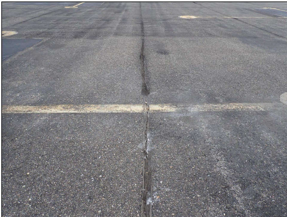
AP-11-08: L&T Cracking
