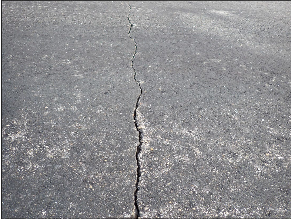
RW11-01-49: L&T Cracking
